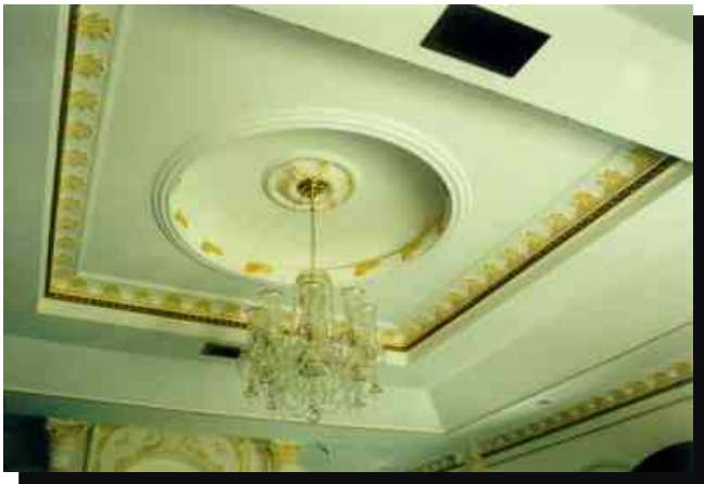
Ceiling Detail Treatment including 'Perennial' crown, 'Perennial' medallion, and 'Versailles with Leaf' panel moulding.
